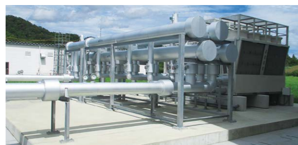
Electric chiller (Ayabe Engineering Plastics Co., Ltd.)
